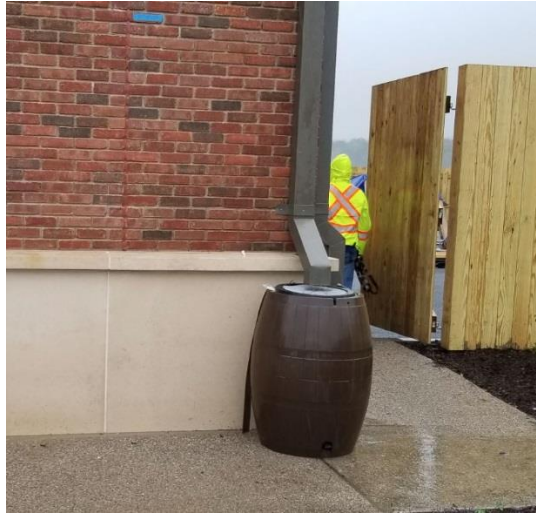
Cistern for collection of rooftop runoff (Photo: New Baltimore Welcome Center, Greene County, NY)
